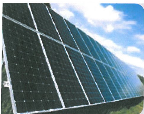
PVSolar field array – National Botanic Garden of Wales
